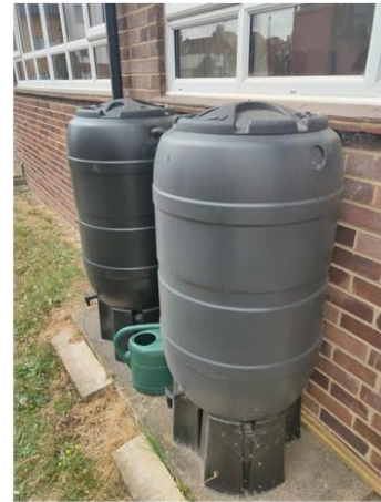
Water butts installed to conserve water for the raised beds
